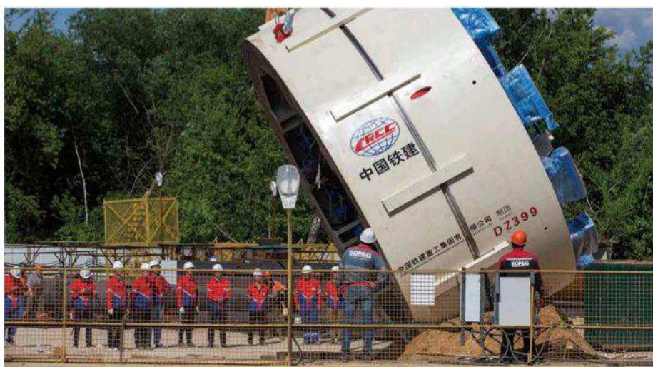
Workers from the China Railway Construction Corporation operate a crane at a subway construction site in Moscow on June 4
